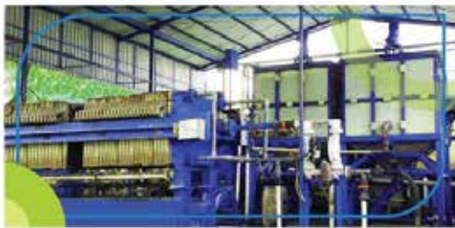
■ Waste Water Treatment Plan
